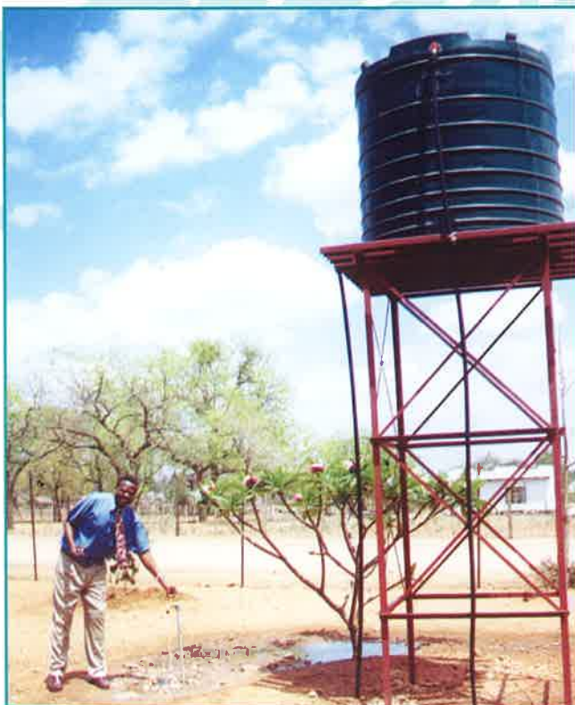
Borehole and tank at a Mahlale school
